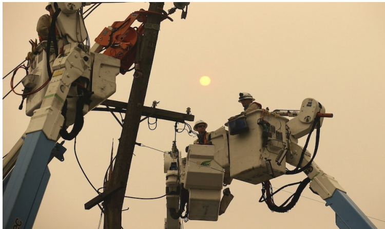
Pacific Gas & Electric crews work to restore power lines in Paradise, Calif., on Nov. 9, 2019. (AP Photo/Rich Pedroncelli, File)
