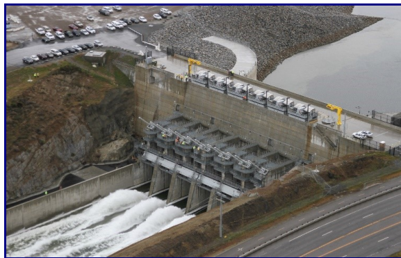
Folsom Dam and Reservoir is being raised 3.5 feet in a $16 million project to allow more water inflows during storms and increase water storage. (Photo courtesy of Sacramento Area Flood Control Agency (SAFCA))
