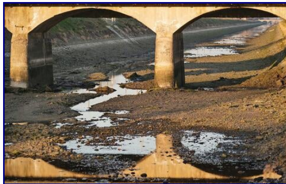
Drying rivers can impact the stability of infrastructure, including bridges. (MikeDot/iStock/Getty)
