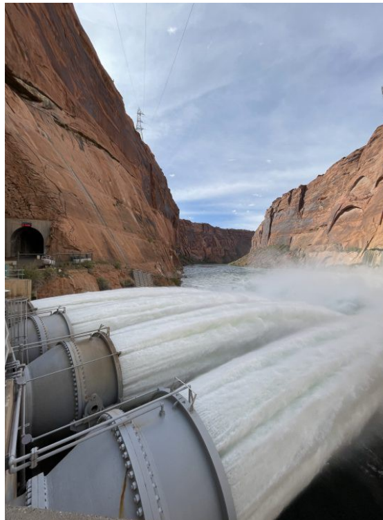
April 24, 2023 – Glen Canyon Dam High-Flow Release. The pipes shown are part of the river outlet Works. (U.S. Bureau of Reclamation)
