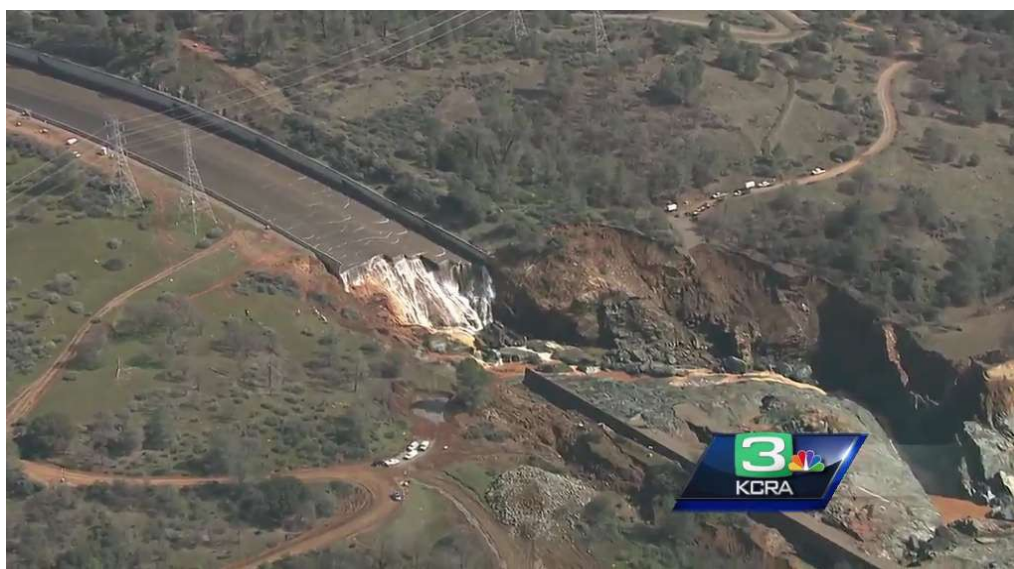
Here is a February 27 picture of the damage to the main spillway
