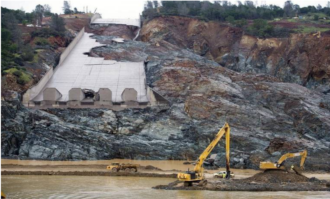
Excavators dredge along the edge of the diversion pool below the spillway at Oroville Dam on April 6. Randy Pench rpench@sacbee.com
